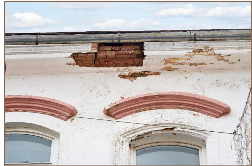
Figure 14. Example of a deteriorated stone cornice. 19
