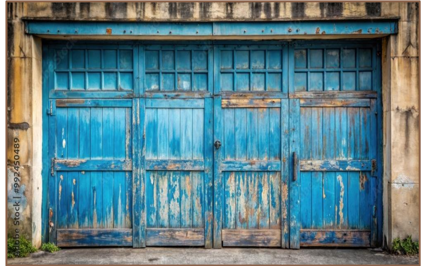
Figure 9. Example of slightly deteriorated woods door with peeling paint. 13
