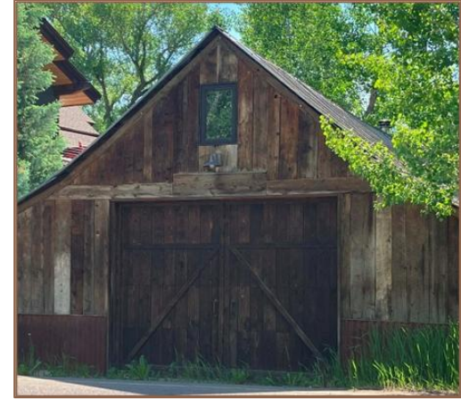
Photograph 14. Barn with non-historic picture window above doors.
