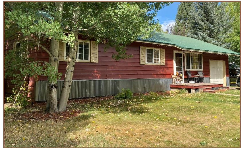
Figure 13. Example of corrugated steel siding over wood lap siding for the purposes of weatherproofing. The corrugated steel siding covering material is removable. 18
