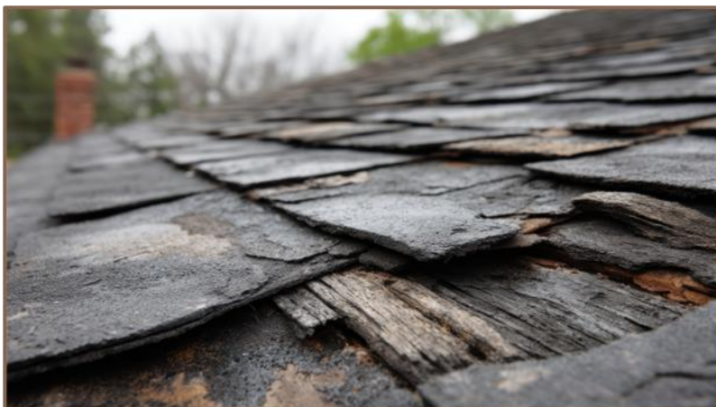
Figure 7. Example of a deteriorating roof. 10
