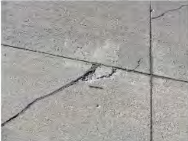
Joint Spalling (Sample Unit No. 11)
