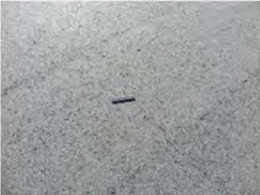
Long. and Trans. Cracking (Sample Unit No. 02)
