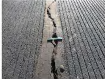
Long. and Trans. Cracking (Sample Unit No. 18)
