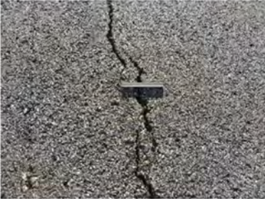
Long. and Trans. Cracking (Sample Unit No. 06)
