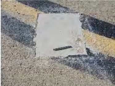
Small Patching (Sample Unit No. 01)
