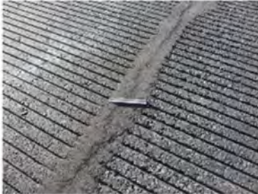
Long. and Trans. Cracking (Sample Unit No. 10)
