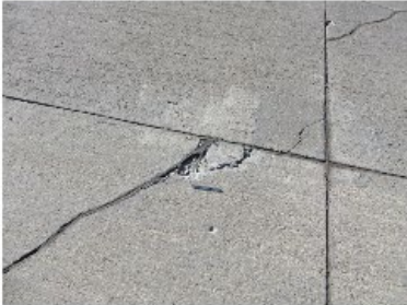
Joint Spalling (Sample Unit No. 11)
