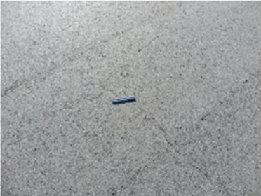
Long. and Trans. Cracking (Sample Unit No. 02)
