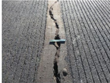
Long. and Trans. Cracking (Sample Unit No. 18)
