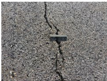
Long. and Trans. Cracking (Sample Unit No. 06)
