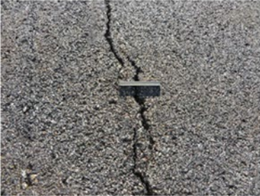
Long. and Trans. Cracking (Sample Unit No. 06)
