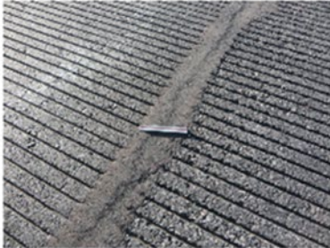
Long. and Trans. Cracking (Sample Unit No. 10)
